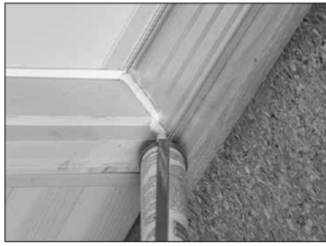
FIGURES 24 and 25: Caulk the sill crown and the top of the sill.
