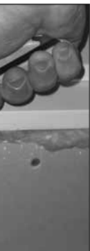
FIGURE 23: Insulate between the jamb and the wall studs all around the door.
